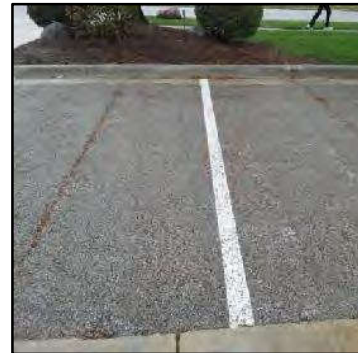
Pervious concrete within a parking lot with debris beginning to accumulate on the surface. Credit: Chagrin River Watershed Partners, Inc.
